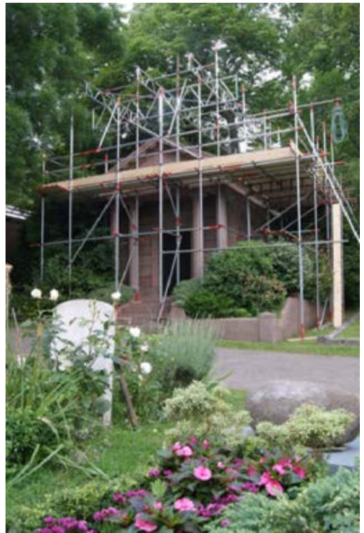
Right: Pocklington Mausoleum awaiting repairs
